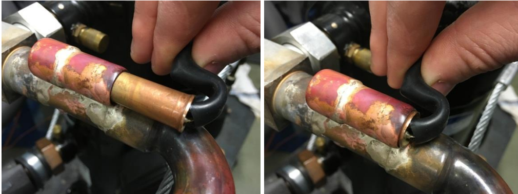
Figure 5: Short copper pipe brazed on the discharge line to hold the DTC valve bulb
