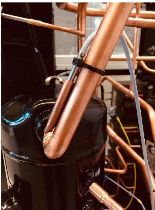
Figure 1: Discharge line temperature sensor
