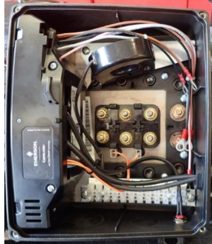
Figure 7: T-box internal view Stream-N
