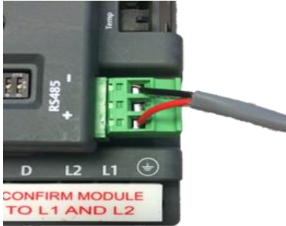
Figure 7: CoreSense Modbus Connections
