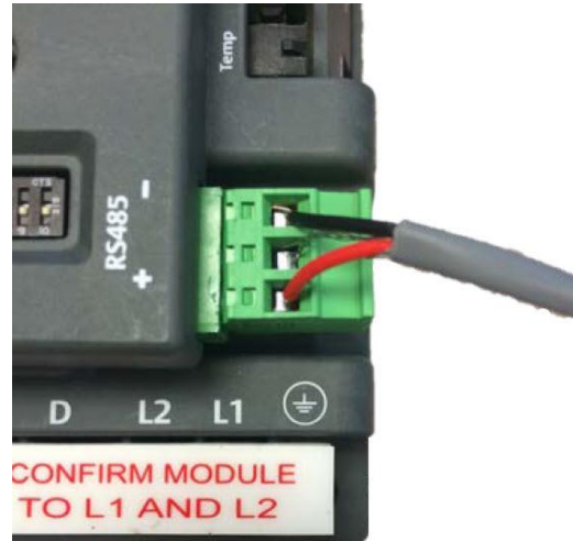
Fig. 6 - CoreSense™ Diagnostics Modbus Connection
