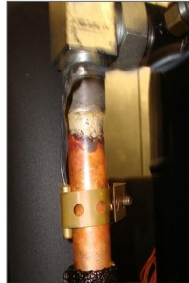
Figure 31 - Discharge Line Thermistor
